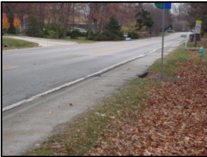
Figure 1. Dangerous shoulder on Hoover Road.
